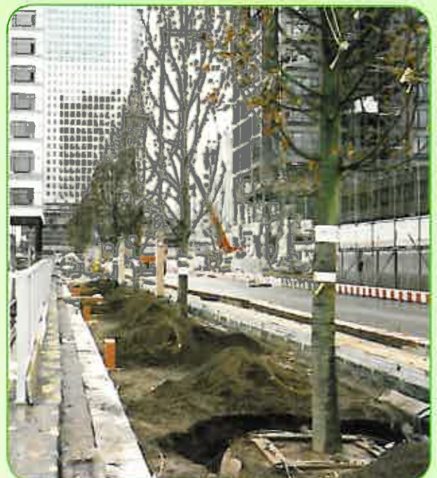
Note the visual effect. A line of 10 m tall trees all anchored with the Platipus tree anchoring system.
